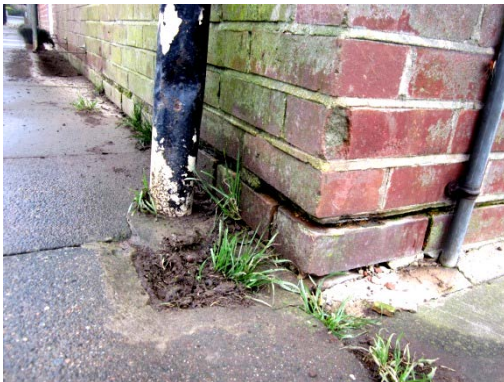
Damaged pointing requires rectification
