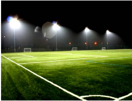
Example of efficient floodlights
