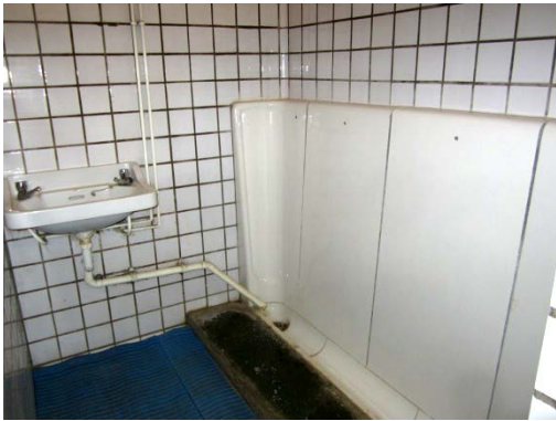
No water supply to urinals
