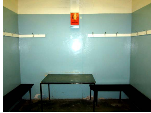
Undersized changing rooms
