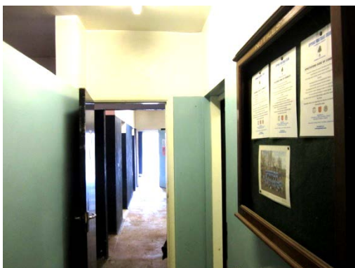
Inadequate emergency provision
