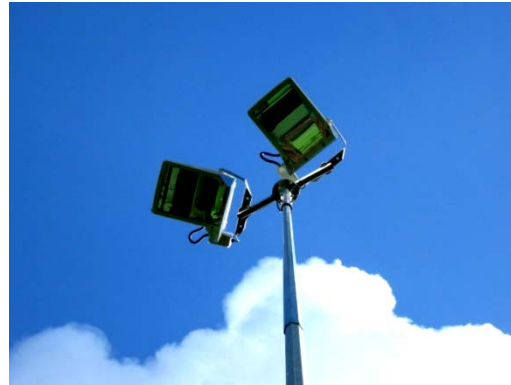
Example of floodlight mast mounted with two luminaires c/w 2kW lamps / fitting
