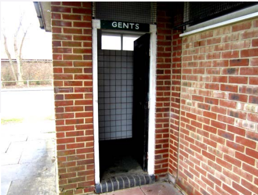
Inadequate access to external WC's
