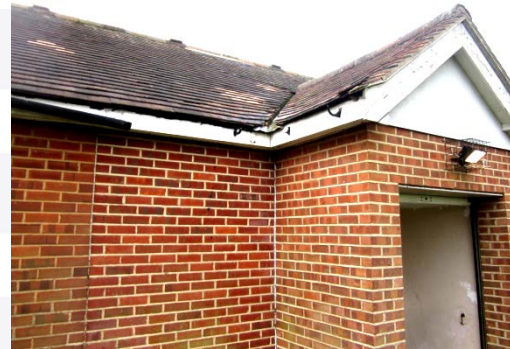
Damaged guttering requires rectification
